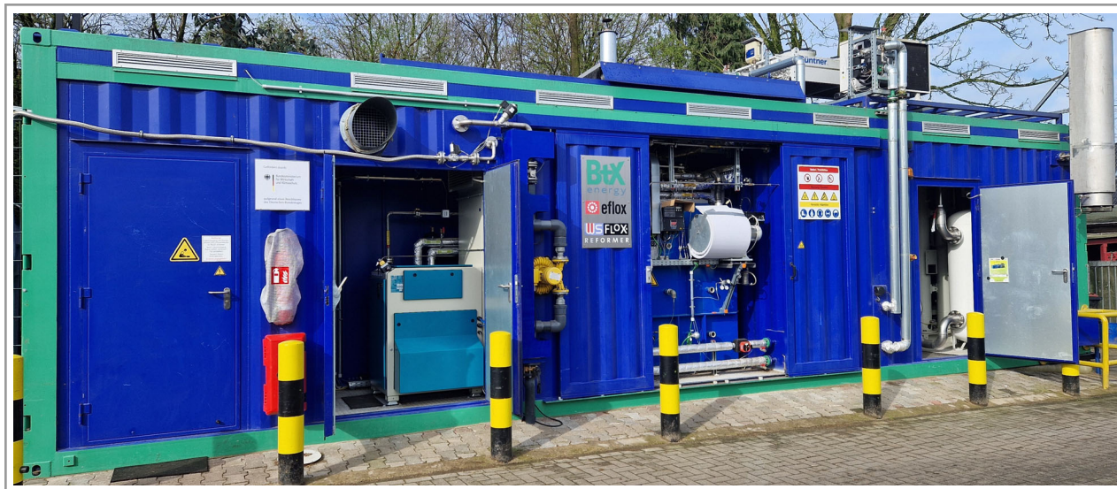
Figure 1. Biogas steam reforming plant of the company BtX energy GmbH, installed in Krefeld.
