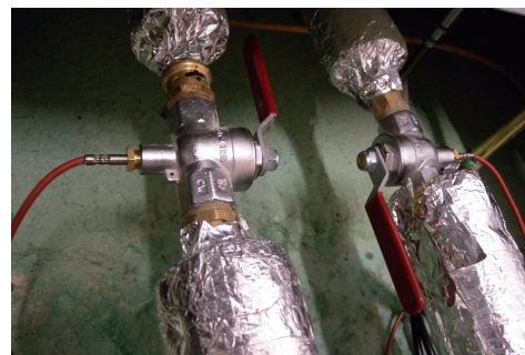
(b) Temperature sensors, cooling supply for façade ventilation unit
