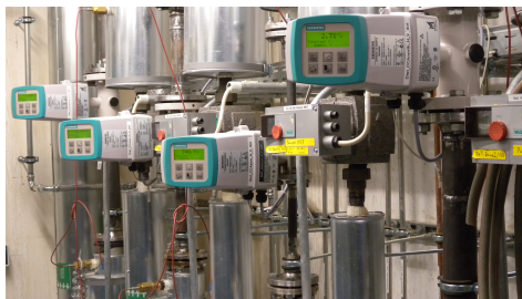
(a) Magnetic-inductive volume flow sensors, different concrete core activation zones
