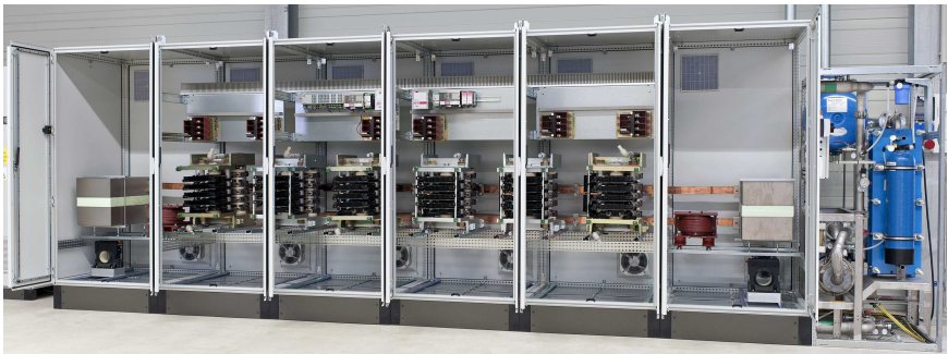
Figure 5.5: DC-DC converter during an early construction phase
