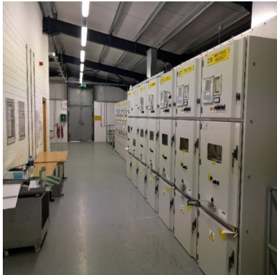
Figure 8 38/20 kV 'Burnwood' GIS Substation in ESB networks
