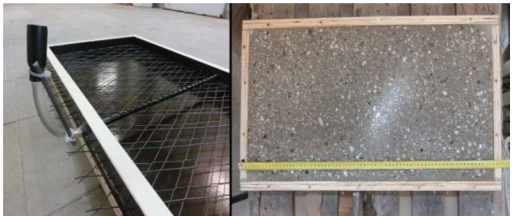
Figure 3. Installed liquid junction (left), concrete base plate (right) according to Henkel (2014).
