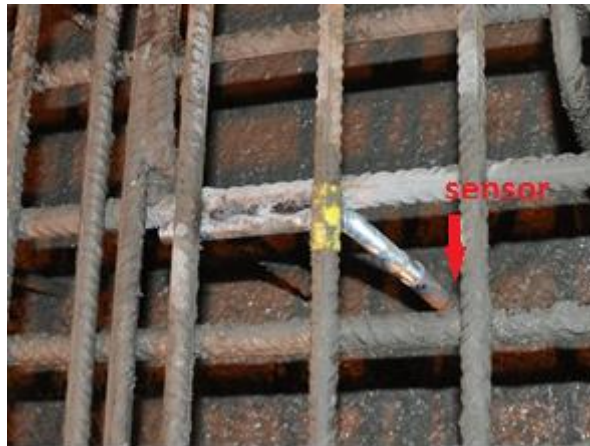
Figure 4-6: Photograph of an ultrasonic transducer mounted at a bridge construction site before casting (Photo: neostrain S. A.).
