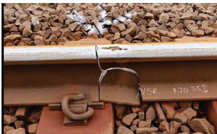
Figure 5: Rail break with residual electrical contact
