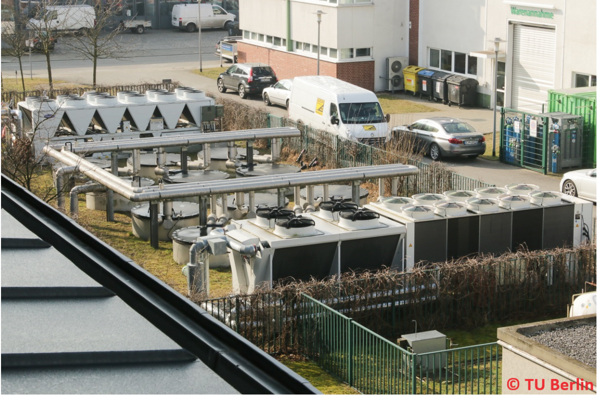
Figure 4.11: A photograph of the cooling supply system investigated in case study two. The two compression chillers and the ice storage tanks are visible [EnBA-M, 2018].
