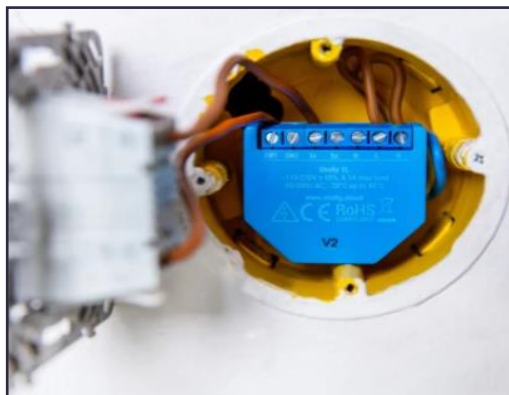
Figure 4: Shelly smart light switch
