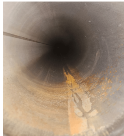
Figure 6.29: Internal surface aspect of the DN250 - 16 m long mild steel chamber before the first heating cycle was applied. Patches of hydroxides and oxides cover the surface.
