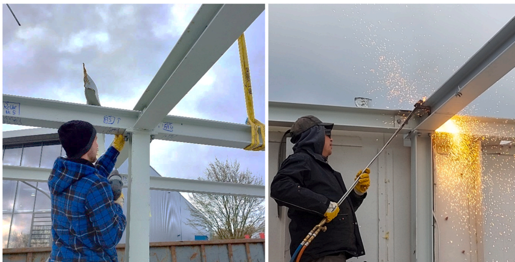
Fig. 5. Careful deconstruction of steel beams: Loosening bolted connections (left) and thermally cutting through beams (right).
