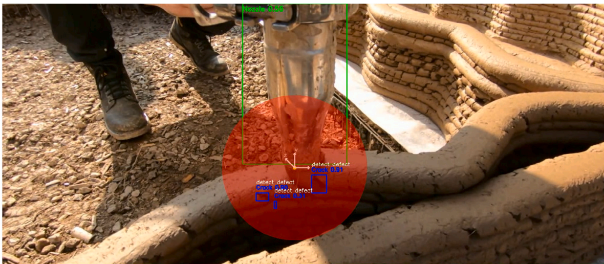
Fig. 11. Live inference frames showing integration of nozzle tracking, crack segmentation, and dynamic ROI filtering in real-time during printing.
