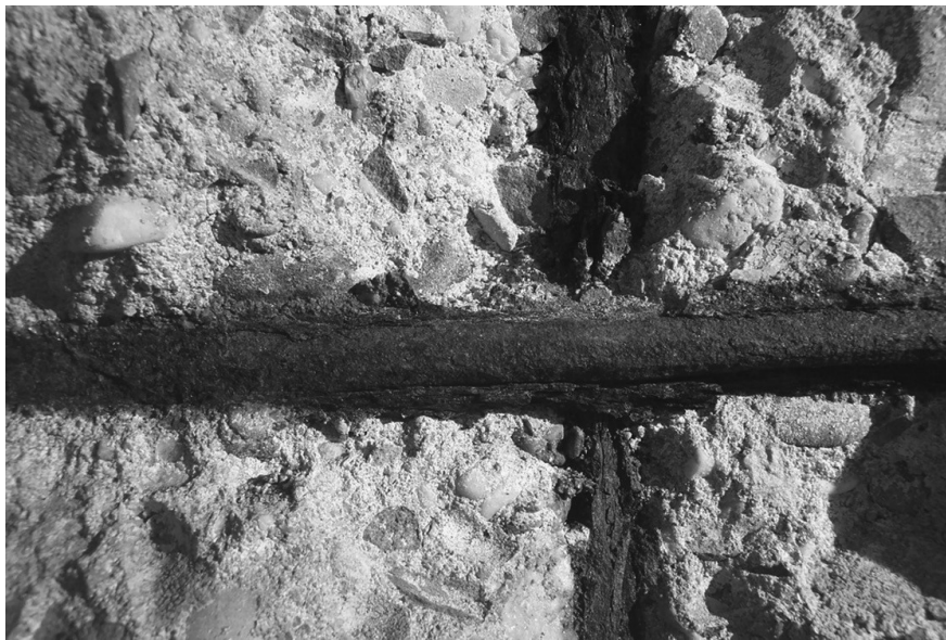
Figure 2-7: Example of a steel reinforcement rebar with visible cross-sectional loss due to carbonation-based corrosion [15].
