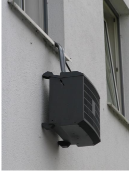
(a) air-conditioning unit on a wall
