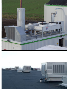
(b) air-conditioning units on a roof
