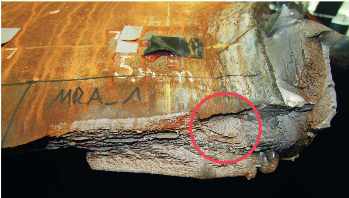
Figure 7.36.: Probable initiation site of failure. The fan-like structure in the HAZ of the weld seam, marked by the red circle, is the suspected crack origin.
