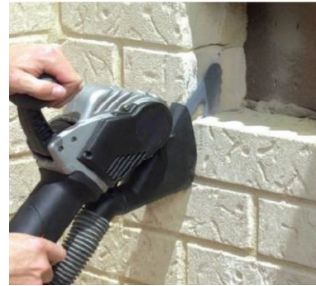
Figure 14 – Wall cutters can be used for dismantling plaster, brick and mortar walls
