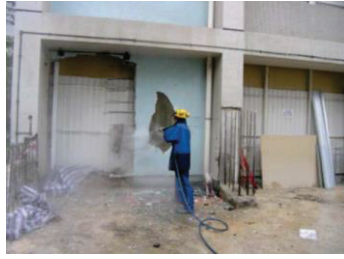
Figure 12 – High pressure water jetting machines can be used for removing deteriorated concrete and tiles
